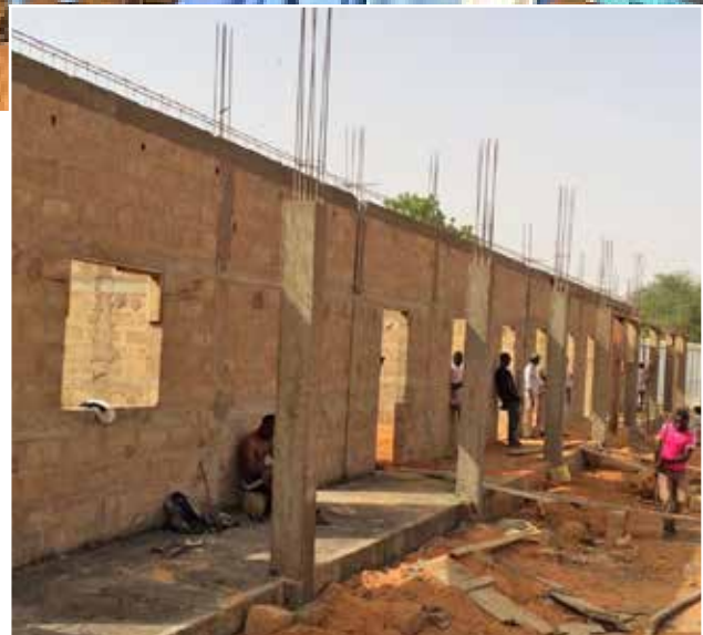
Four classrooms for secondary school students are under construction at the Niamey School for the deaf.
